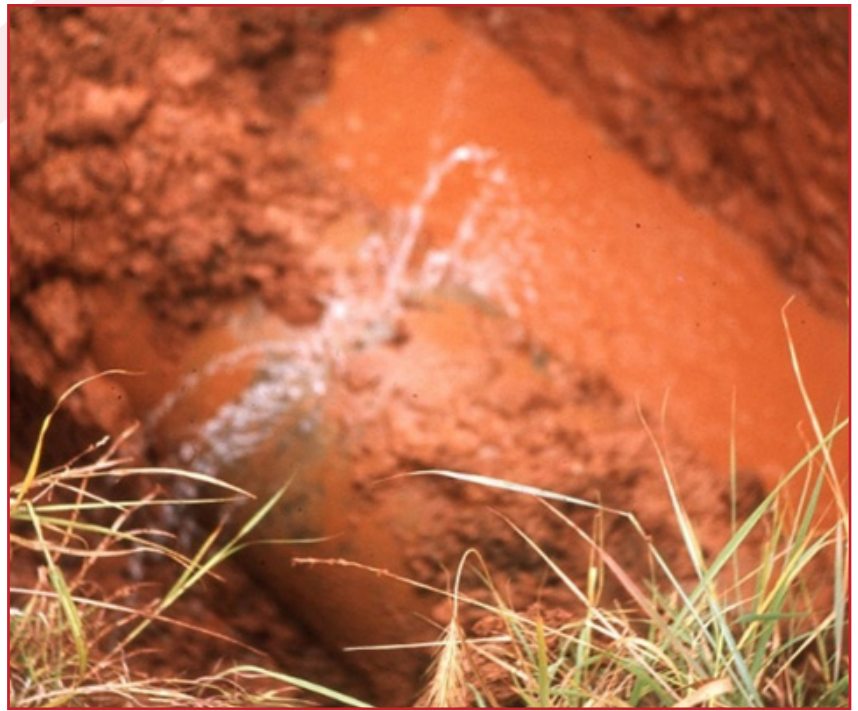
Broken Back Crack in Concrete Pipe
