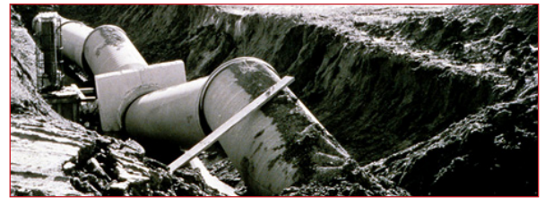
Flotation of Pipe Before Backfilling Completed
